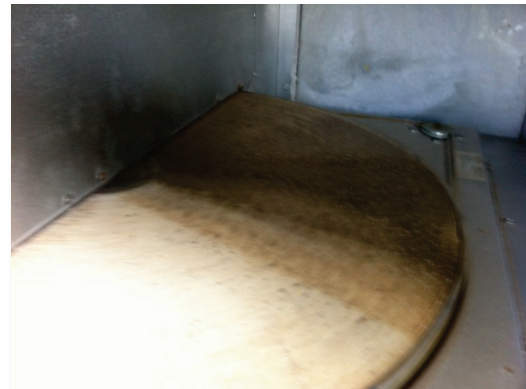
Figure 35 - AHU Energy Recovery Wheel
