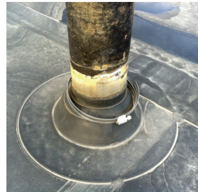
Figure 8 – Vent Penetration (note untightened band clamp)
