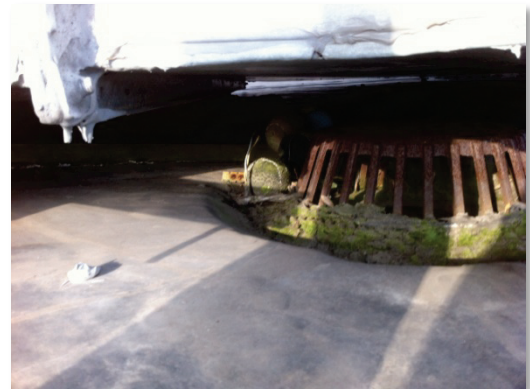
Figure 38 – Clogged Scupper under AHU-4
