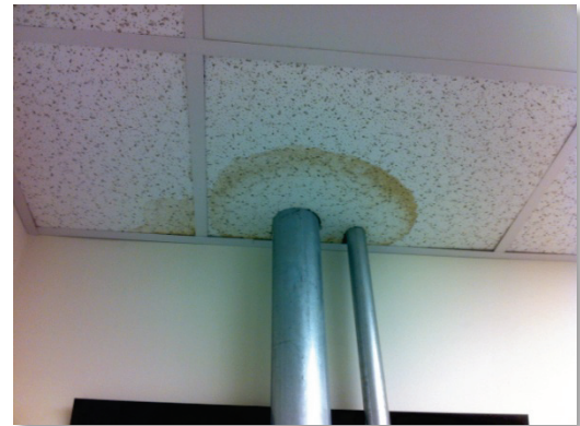
Figure 17 – Water Stains around Electrical Panel Conduit
