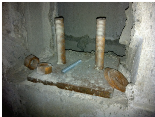
Figure 37 – CMU Wall Plate with Missing Bolted Connections
