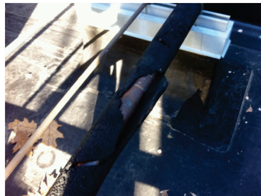
Figure 25 – Deteriorated Condenser Pipe Insulation
