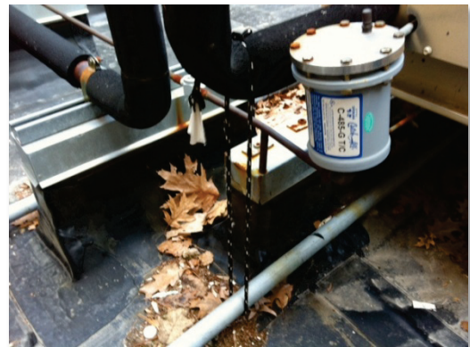
Figure 27 – Shoelace Tied to Condensate Pipe as Electrical Conduit Support
