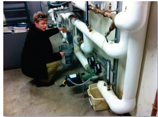
Figure 28 – Leaking Hydronic Pumps with Buckets
