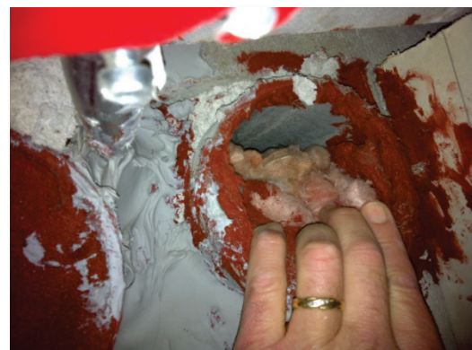
Figure 41 – Unsealed Conduit in Fire Barrier Wall
