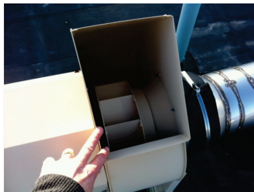
Figure 30 – Lab Exhaust Ventilator w/ no Guard
