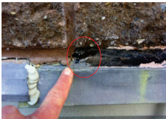
Figure 39 – Gap in Masonry Wall Flashing Joint
