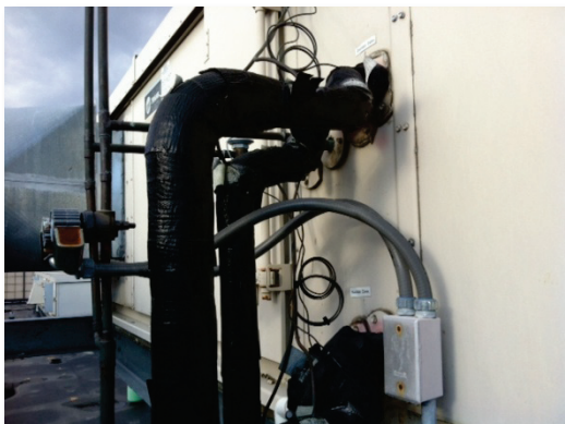
Figure 26 – Duct Tape on Deteriorated Pipe Insulation
