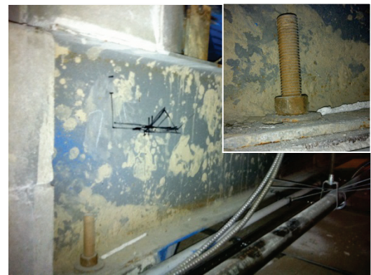
Figure 36 – Structural Beam with Loose Bolted Flange Connection and no Fireproofing
